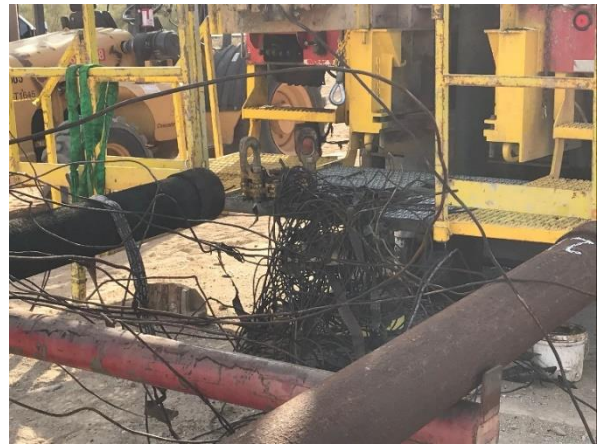
Transducer wire that was removed from the well
