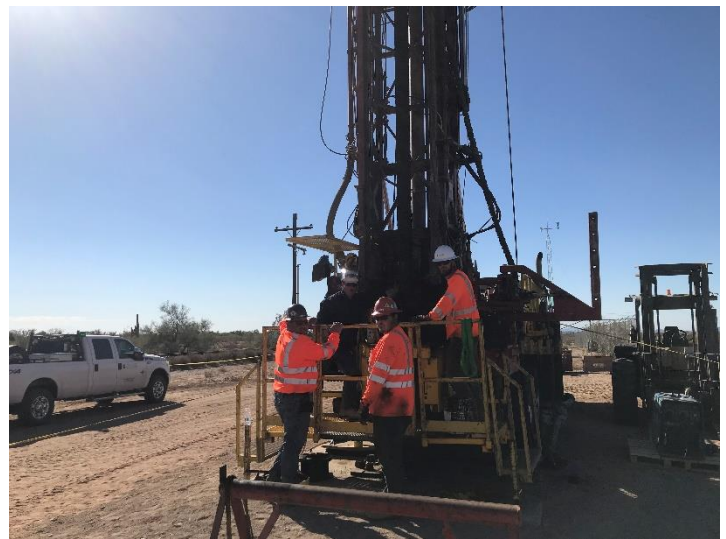
Crew having a safety discussion on the work platform of the drill
